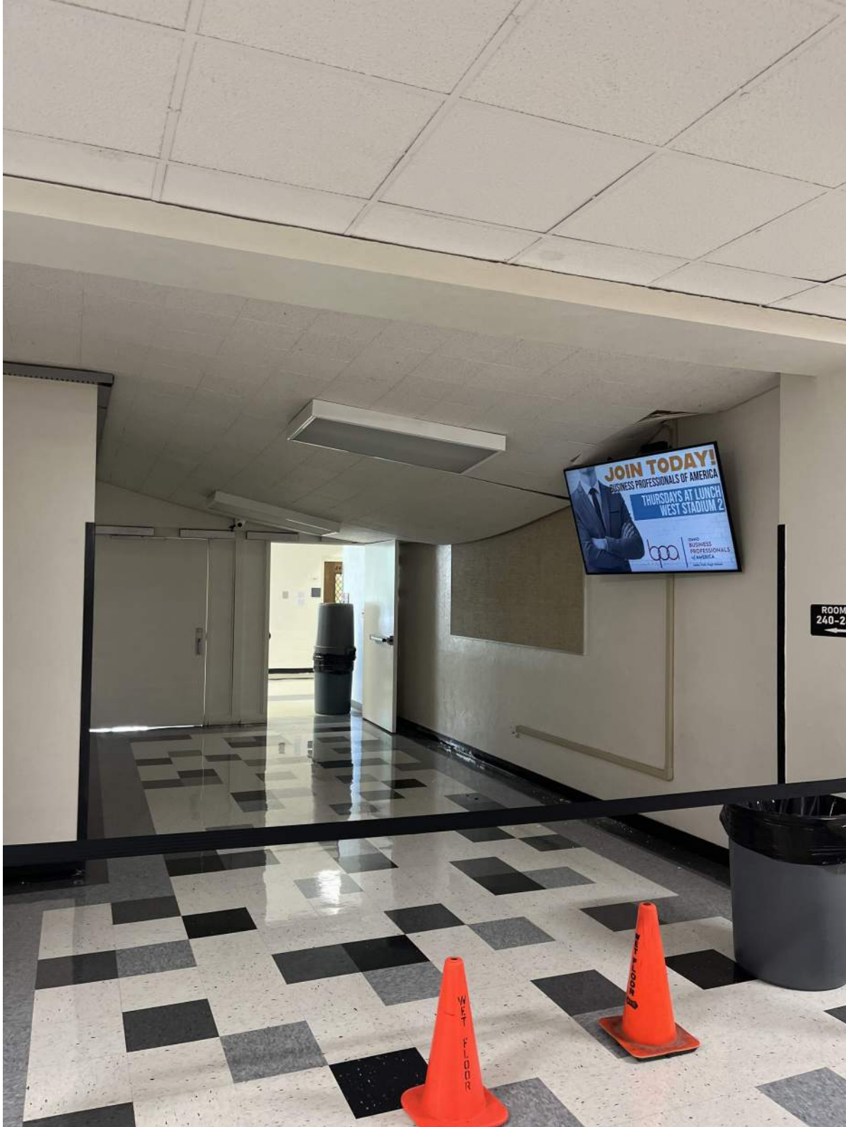
Photo #1 - Collapsed ceiling in hallway
