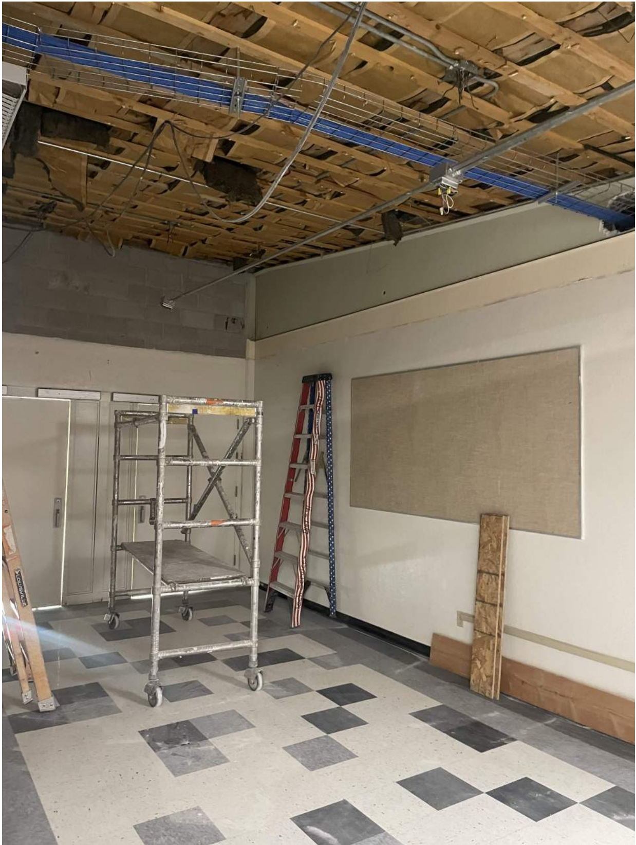
Photo #2 - Area where ceiling collapsed, after removal
